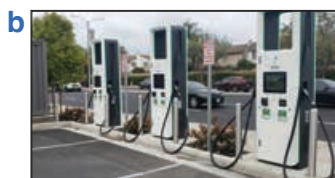
b charging station
